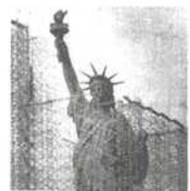
RISE — Steel scaffolding rises around the Statue of Liberty in New York Harbor. The framework is in preparation for a $30 million renovation project.
