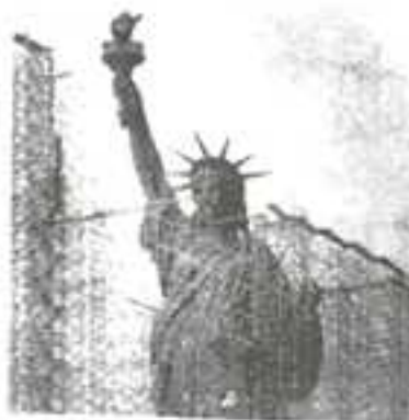
RISING —Steel scaffolding rises around the Statue of Liberty in New York Harbor. The framework is in preparation for a $30 million renovation project.
